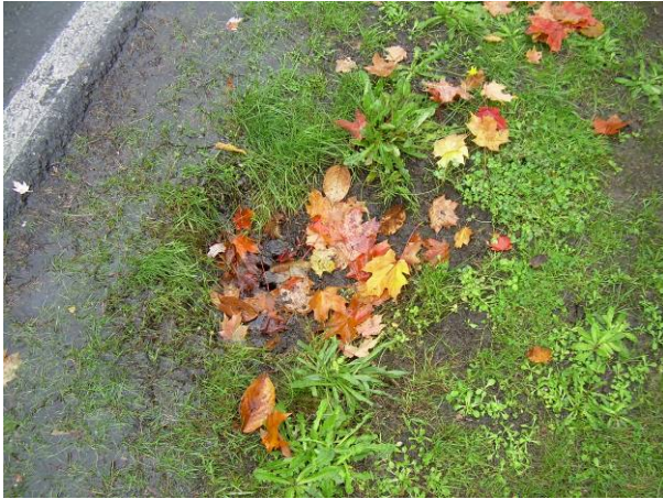
Figure A-3 Existing pot drain clogged with leaves and no flow path into the structure
