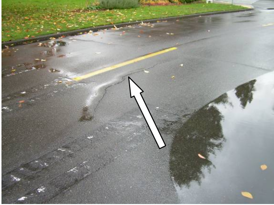
Figure D-4 Roadway settlement in the northbound lane
