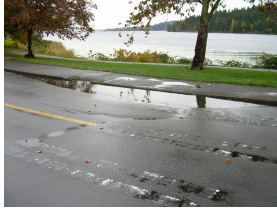
Figure D-5 Ponding caused by the settlement in the roadway
