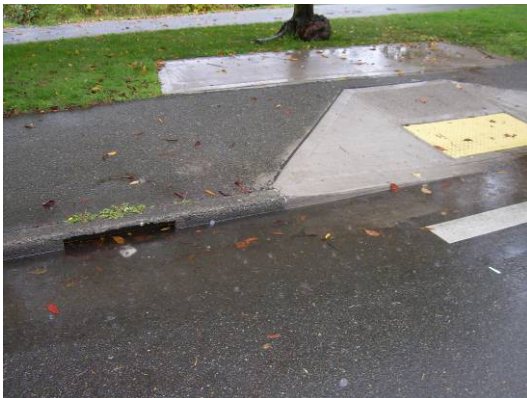
Figure D-3 Clogged drain near the north ADA ramp
