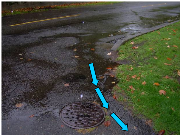
Figure A-2 Storm water sheet flows down the driveway to the boat park
