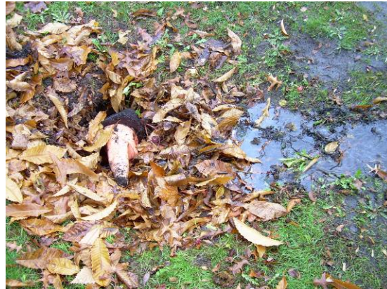
Figure B-3 Location of missing pot drain
