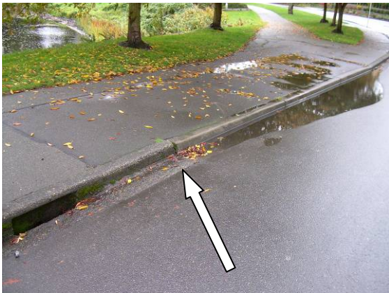
Figure D-6 Undulations in the roadway preventing runoff to drain
